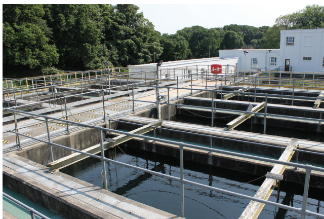
Clarifiers at Handois water treatment works
