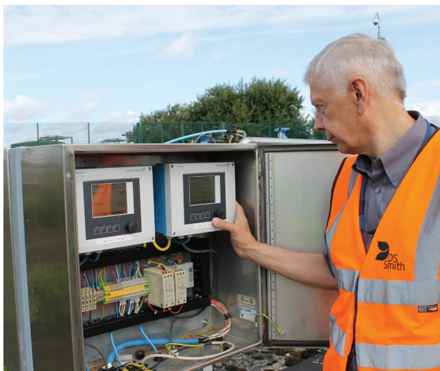
Two pH transmitters are required for regulatory purposes.
