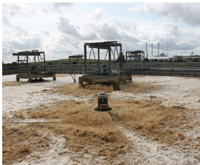
Waste effluent is re-oxygenated before being discharged into the Swale estuary.
