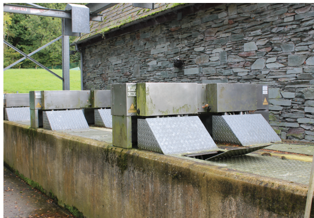
Housing for the UV lamps
